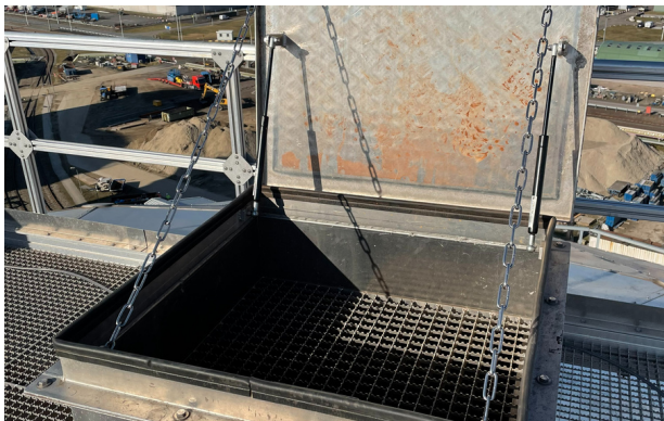
Elevated Manway Hatch
