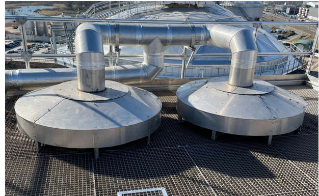
OCU Ventilation Piping (Pressure + Relieve)
