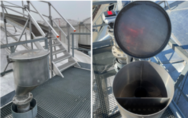
Hatch Covered Sample Point
